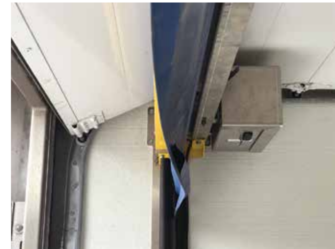
The yellow bar is just 2 1/2 inches below the rest position of the raised roll-up door. The motor operator is hung behind the mandrel.
