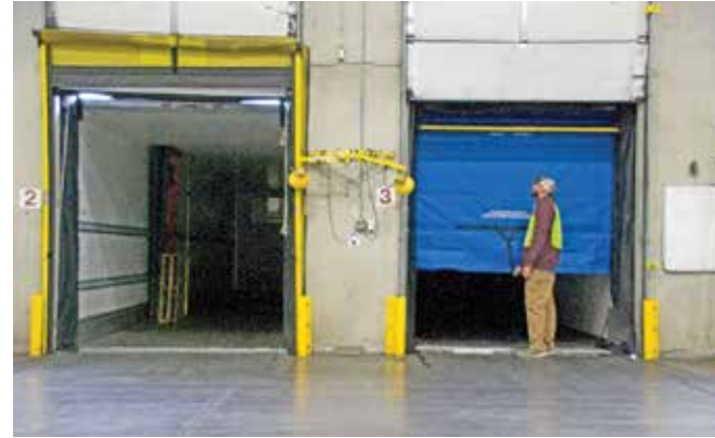
The Kool Shield is shown deployed at a loading dock.
